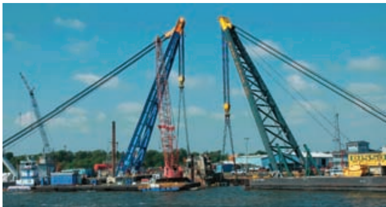
The 600 ton capacity D/B BIG T, owned by T&T Marine Salvage of Galveston, Texas, and the 700 ton capacity D/B Cappy Bisso, owned by Bisso Marine of Houston, Texas, were used to make a tandem lift of a 105' sunken tugboat in Port Arthur, Texas.
